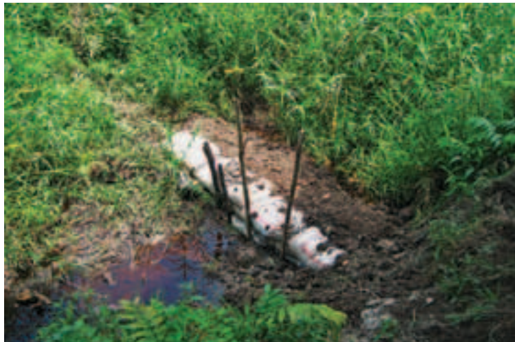
FIGURE 14 Small ditch blocked with sandbags and soil.
