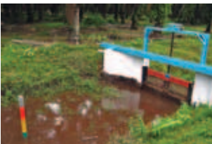
Figure 7: An example of a water control structure.
