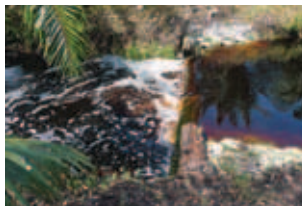
Figure 8: One weir installed at every 20cm drop in water level to enable water retention along collection drains.
